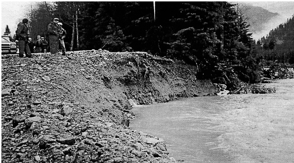
Figure 6-1: Eroding Road Bank along the Indian River, looking upstream
